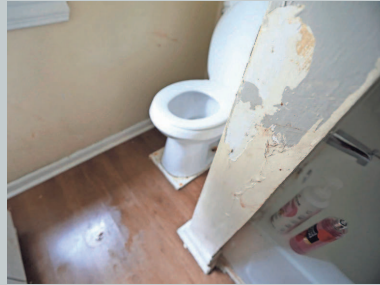
Robinson said on Aug. 6 that on hot days you can smell the mold in the bathroom. She also has problems with the toilet and base of the toilet. A wall between the toilet and bathtub has peeling paint.
