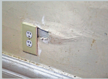
One of the outlets in the living room has part of the bare wall exposed next to it. Robinson said sometimes if the outlet is touched it sparks.
