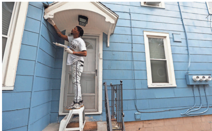
Stephon Hicks, a contractor, caulks an area around the porch roof for the landlord. TINA MACINTYRE-YEE/DEMOCRAT AND CHRONICLE
