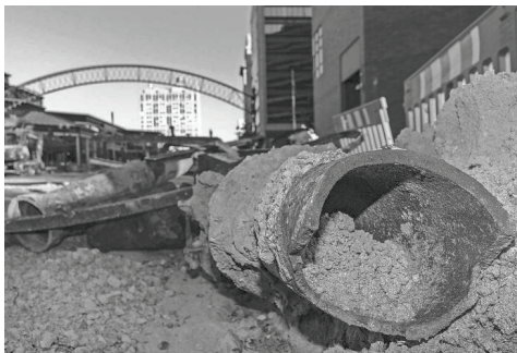
A piece of an old water main lays amid a pile of pipe in downtown Flint, Mich., on Thursday. PHOTOS BY RYAN GARZA/DETROIT FREE PRESS
